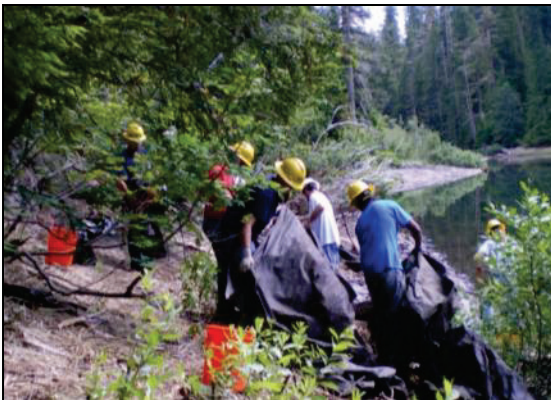
Figure 1. WCC removing landscape fabric at Pine Lake. All bare ground shown in photo was previously occupied by reed canary grass at almost 100% cover. Live willow stakes planted last year are in foreground.
