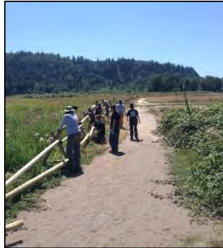
Figure 2. This closure fence is being constructed by YESS crews to provide refugia for all wildlife. To the left of the fence a pollinator hedge is being planted with flowering shrubs (such as elderberry, spiraea, nootka rose, and flowering forbs) to help prevent access. The prairie to the left of the fence will be restored to native prairie in future years.
