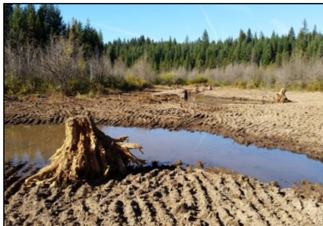
Figure 1. Stump Lake immediately after the ponds had been excavated in the summer of 2014. This wetland area is associated with a PacifiCorp operated reservoir and is being enhanced as a condition of the relicensing of the hydroelectric project.
