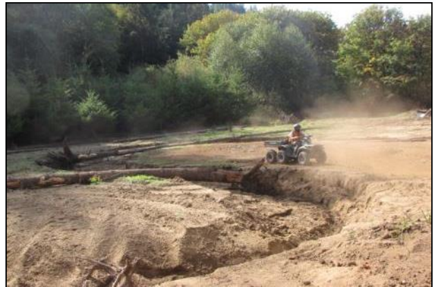
Figure 1. Riparian Restoration. Seedbed preparation. A tined implement pulled behind a modified tractor! The watershed scale Five Mile-Bell riparian restoration project..
