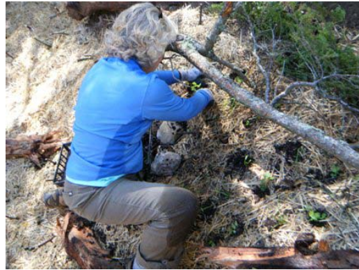
SWP crew leader Linda Rehorst transplanting native plugs into slopes at a new culvert replacement site-GINRA.
