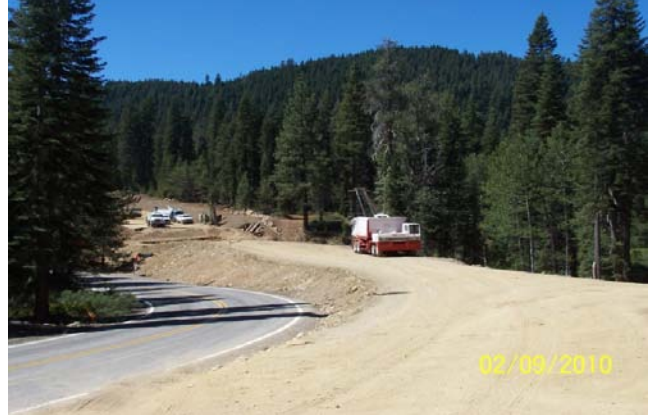
Figure 1. Road and bridge construction to be sown with mountain brome during the fall of 2010.
