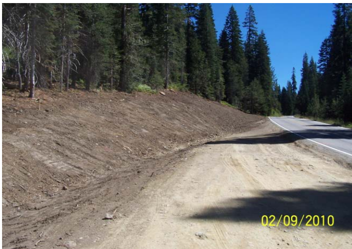
Figure 2. Road construction on Quincy-Oro Highway to be sown with mountain brome during the fall of 2010.
