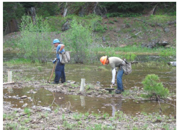
Figure 1. Contractors planting alder, bog birch, dogwood, willow and cottonwood for Clear Creek project.
