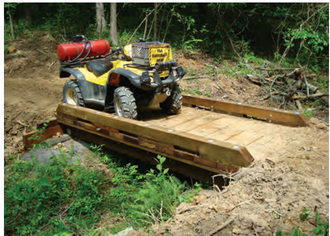
Figure 9—A single-unit timber bridge designed to accommodate all-terrain vehicles, bicycles, and hikers.
