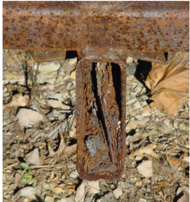
Figure 16—A weathering steel floor beam with corrosion issues in a humid climate.
