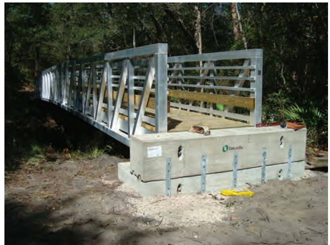
Figure 17—Rub rails installed on an aluminum side truss bridge to protect the railing system.
