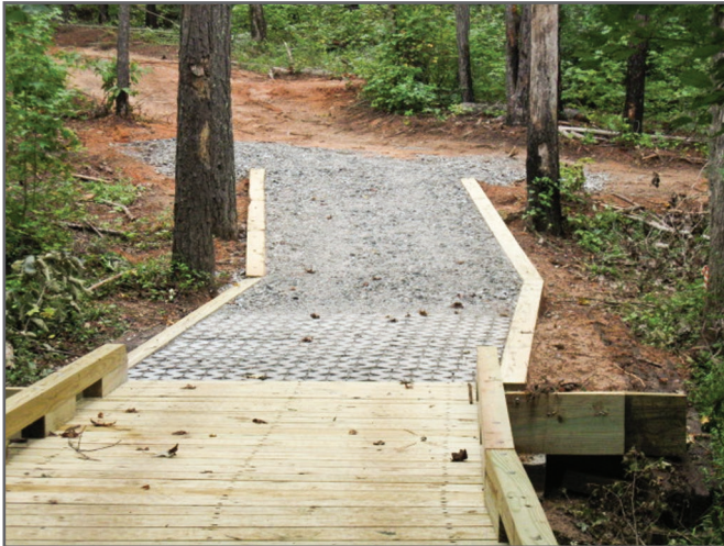
Step 11—Masonry block pavers at the boardwalk approaches provide a firm transition from the trail to the boardwalk and minimize soil settlement.
