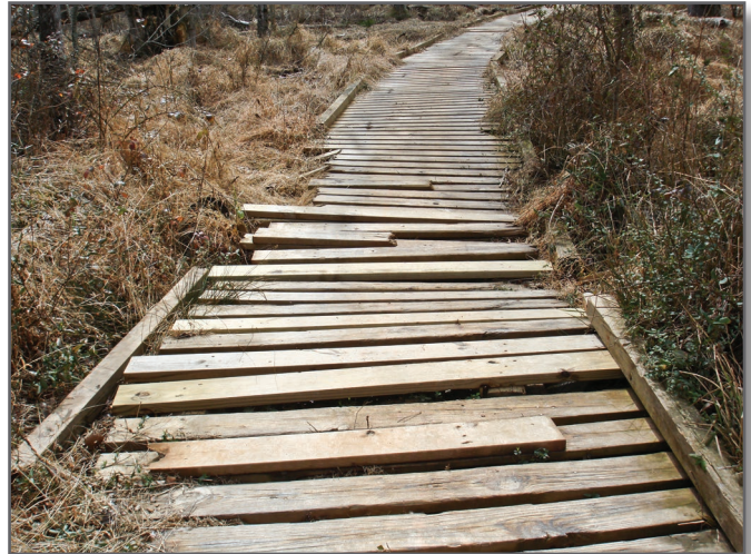
Step 1—The OHV elevated boardwalk is installed during a dry period while accessibility for equipment is good. The first step requires removing the existing deteriorated boardwalk.
