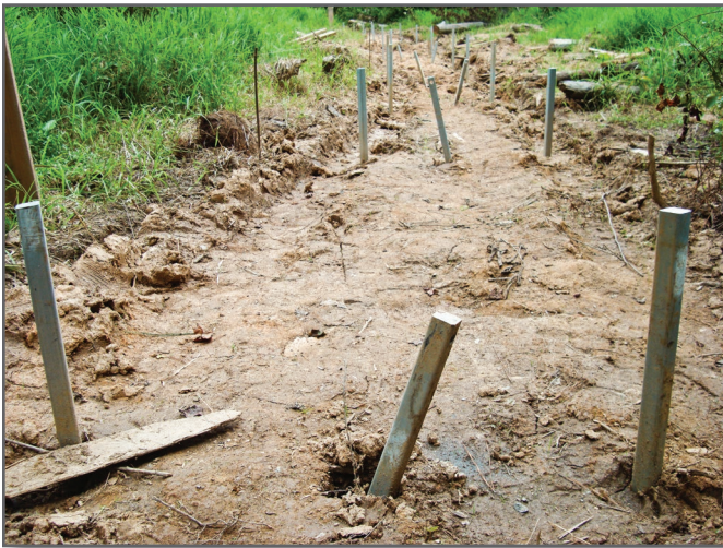
Step 2—Helical piles are installed using a mini-excavator with a special screw head and hydraulics. The contractor installed 90 helical piles at an average depth of 10 feet over 3 long workdays. Helical piles are installed both vertically and at an angle. The direction of the angled piles alternates between bents for lateral bracing purposes.
