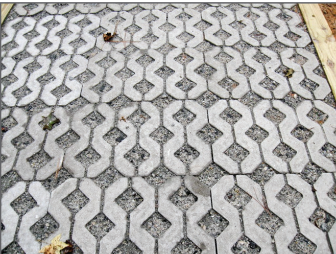
Step 12—A closer view of the Perystone Pavers used in the installation.
