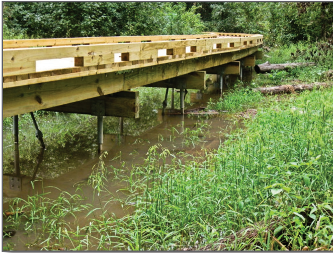
Figure 2—This elevated boardwalk on the Town Creek off-highway vehicle trail system at the Chattahoochee-Oconee National Forest in Georgia is supported by helical piles.
