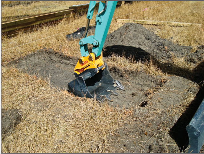
Step 1—A trench 8 feet by 3 feet by 1 to 2 feet (depth depends on the required substructure ground elevation) is excavated to accommodate the wrapped geocell and precast concrete foundation.
