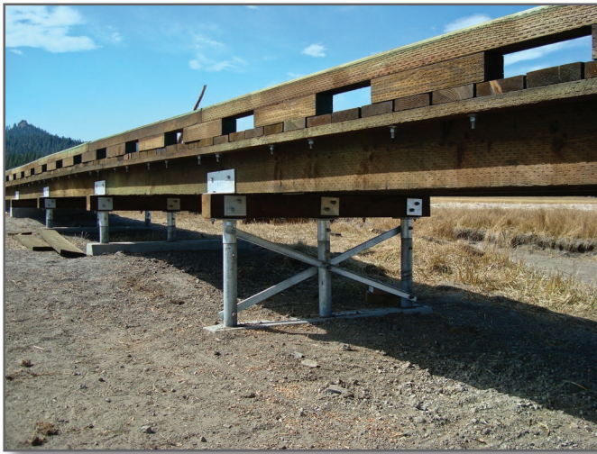
Step 11—The finished structure features curbs with scupper blocks for this ATV/motorcycle trail.
