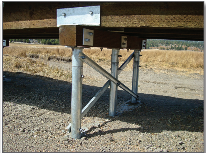
Step 8—Two-inch-wide galvanized steel C-channel cross bracing is added where the structure is 3 feet or higher above the ground.
