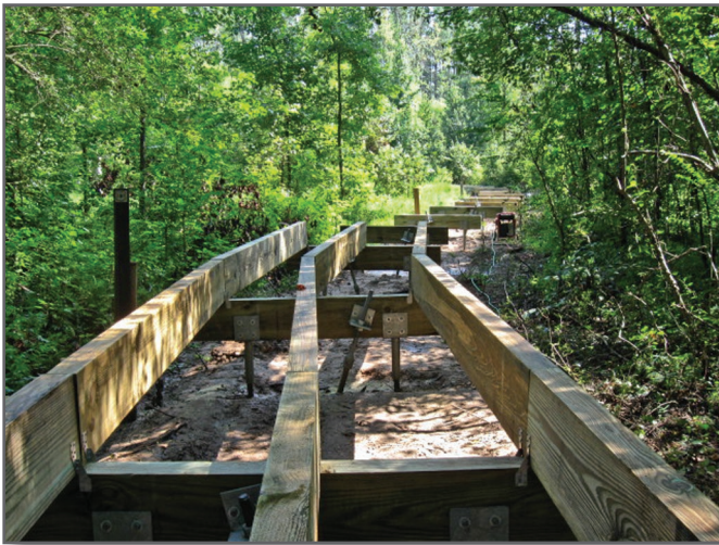
Step 6—Stringers are set in place and attached to the header beams.
