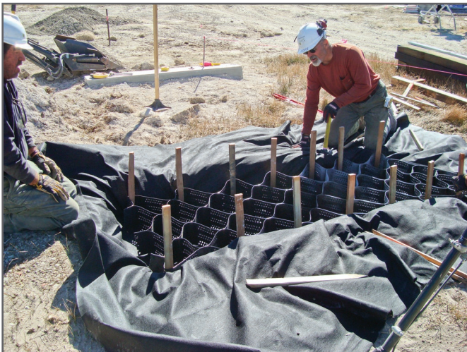
Step 2—Geosynthetic fabric is placed, and the geocell is staked and filled with gravel. Geosynthetic fabric is folded over the top.
