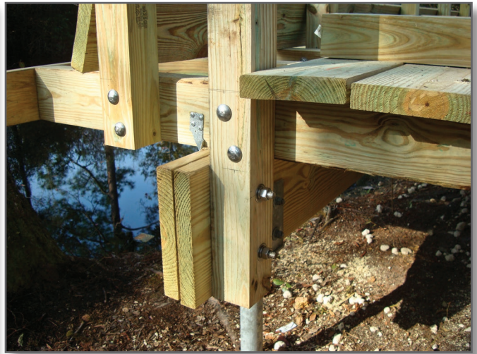
Step 5—The structure is cantilevered 2 feet over the helical piles to allow water to drain off the boardwalk while avoiding the exterior beams. This also allows better access for fishing.
