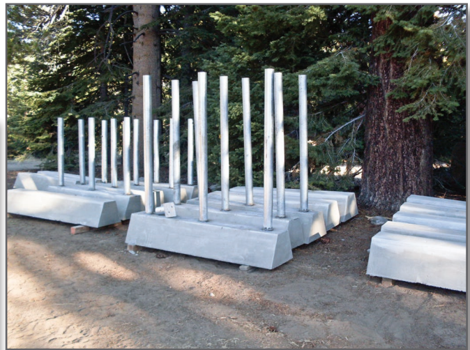
Step 3—The substructure consists of a 6-foot by 18-inch by 12-inch precast concrete foundation. The top of the concrete foundation is 9 inches wide and has a 6-inch by 6-foot by \frac{3}{8} -inch flat steel plate with 7-inch shear studs cast into it. The posts (3-inch diameter galvanized steel pipe with \frac{1}{4} -inch walls) are welded to the steel plate. Rebar hooks embedded in the curb allow the curb to be moved by machine.
