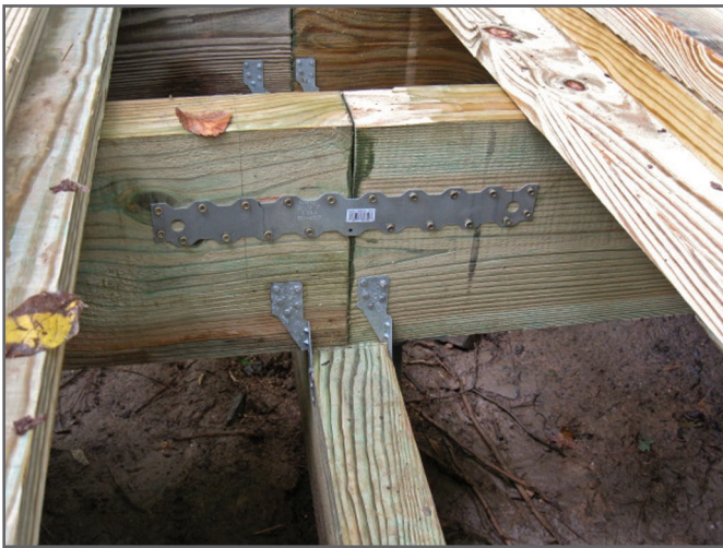
Step 7—Stringers are carefully placed on header beams and Simpson Strong-Tie metal components are used to join members.
