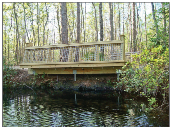
Figure 1—Helical piles support this viewing/fishing platform at the Okefenokee National Wildlife Refuge in Georgia.
