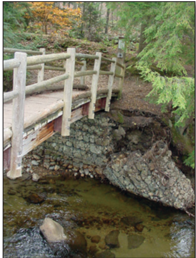
Figure 15—Scour caused by constricting the channel at the bridge site.
