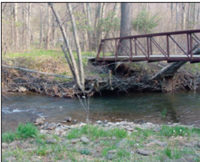
Figure 14—Naturally occurring scour at a bridge.
