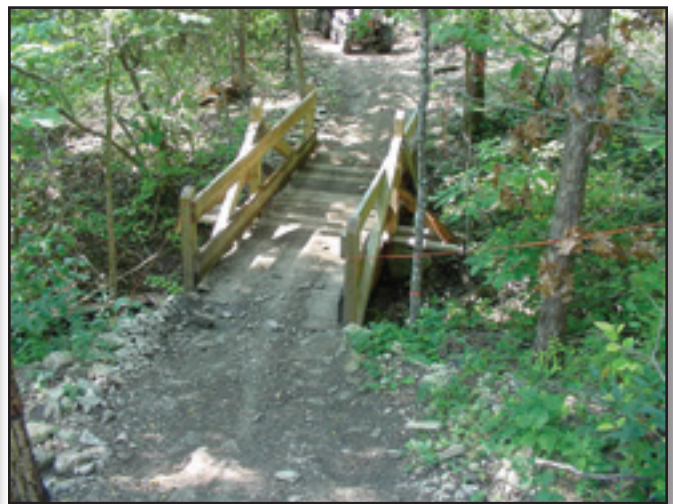
Figure 36—Gravel collects on the deck of this bridge because it is in the low point of a sag curve.
