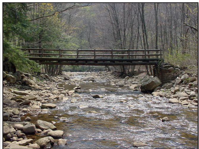
Figure 16—This bridge is on a side stream and in a flood plain. The back-water effect during floods on the main stream has floated this bridge away twice.
