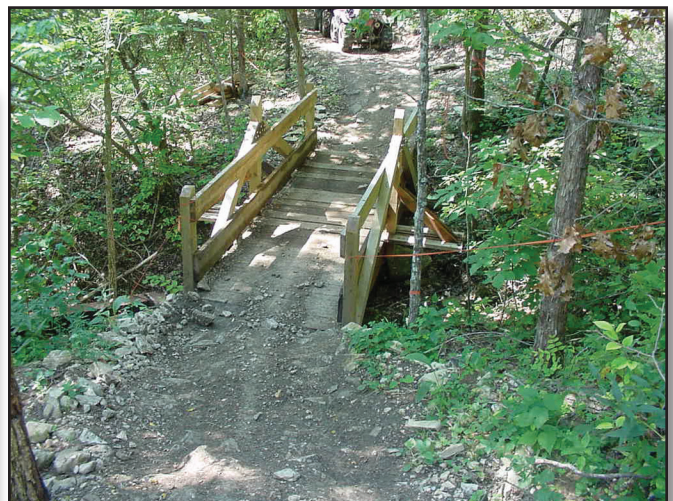
Figure 36—Gravel collects on the deck of this bridge because it is in the low point of a sag curve.
