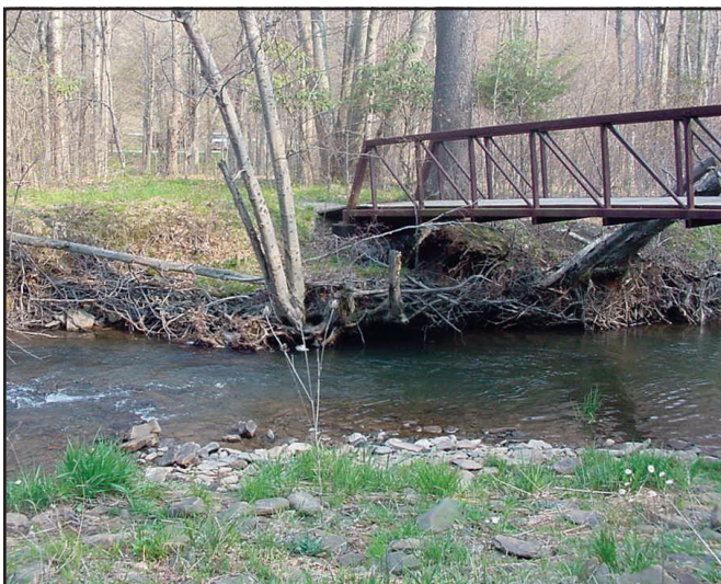
Figure 14—Naturally occurring scour at a bridge.
