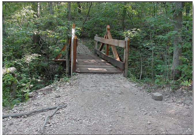
Figure 35—This bridge has a slight grade, allowing water and debris to run off the bridge deck.
