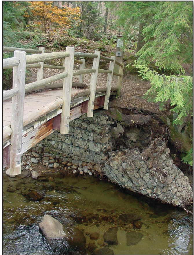
Figure 15—Scour caused by constricting the channel at the bridge site.
