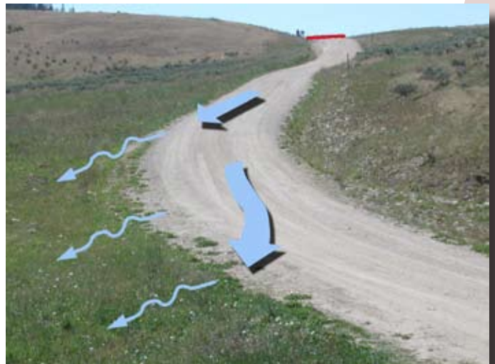
Road surface drainage can be a source of erosion and sediment delivery to streams.
