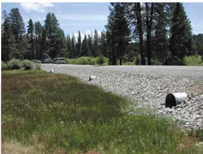
Figure 8—Road riparian restoration techniques use a permeable fill with culverts to cross a meadow.
