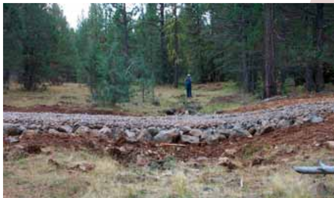
Armored dip on ephemeral stream in Lassen NF, immediately after construction in 2003. Photo by Carolyn Napper.
