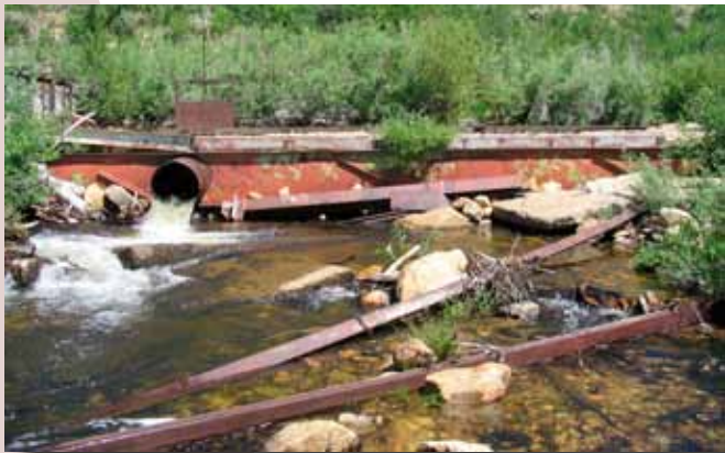
Found-object diversion structure blocking fish and controlling diversion on North Brush Cr, Medicine Bow NF, WY.
