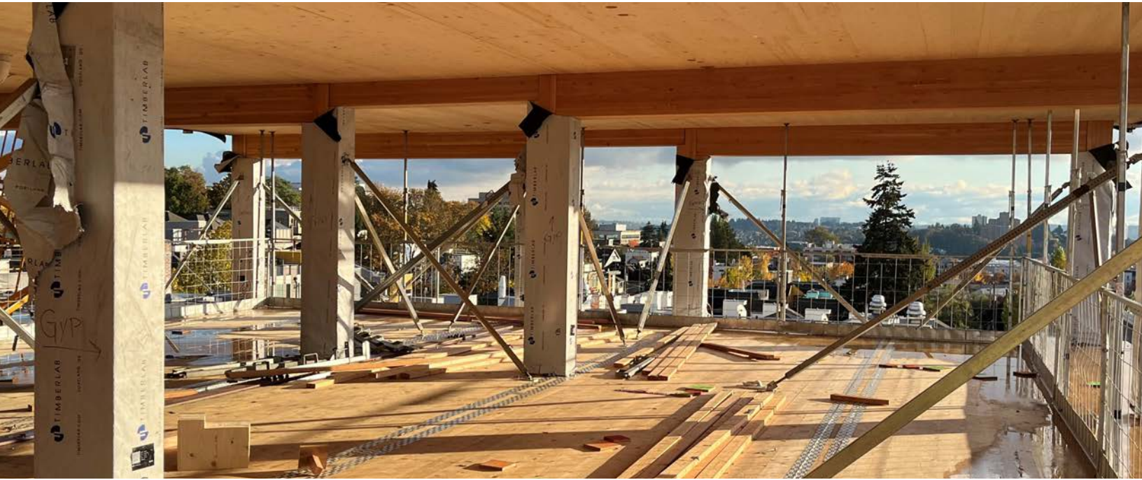
Mass timber superstructure under construction at Heartwood. Courtesy photo by atelierjones, llc.
