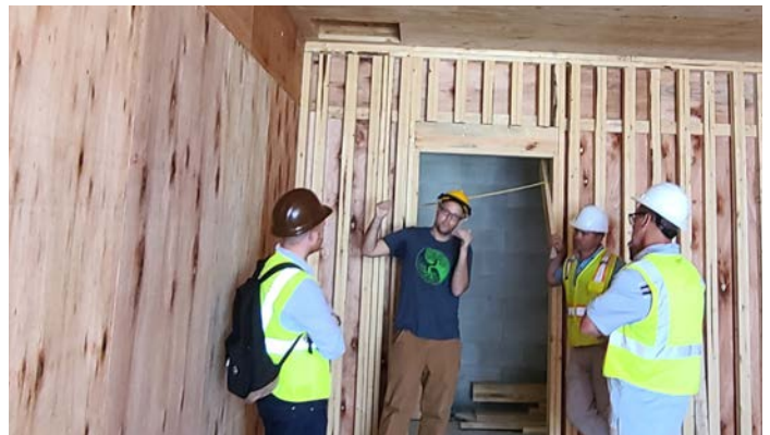
Eastern hemlock CLT installation at 154 Broadway. Courtesy of Innovative Natural Resources Solutions, LLC.
