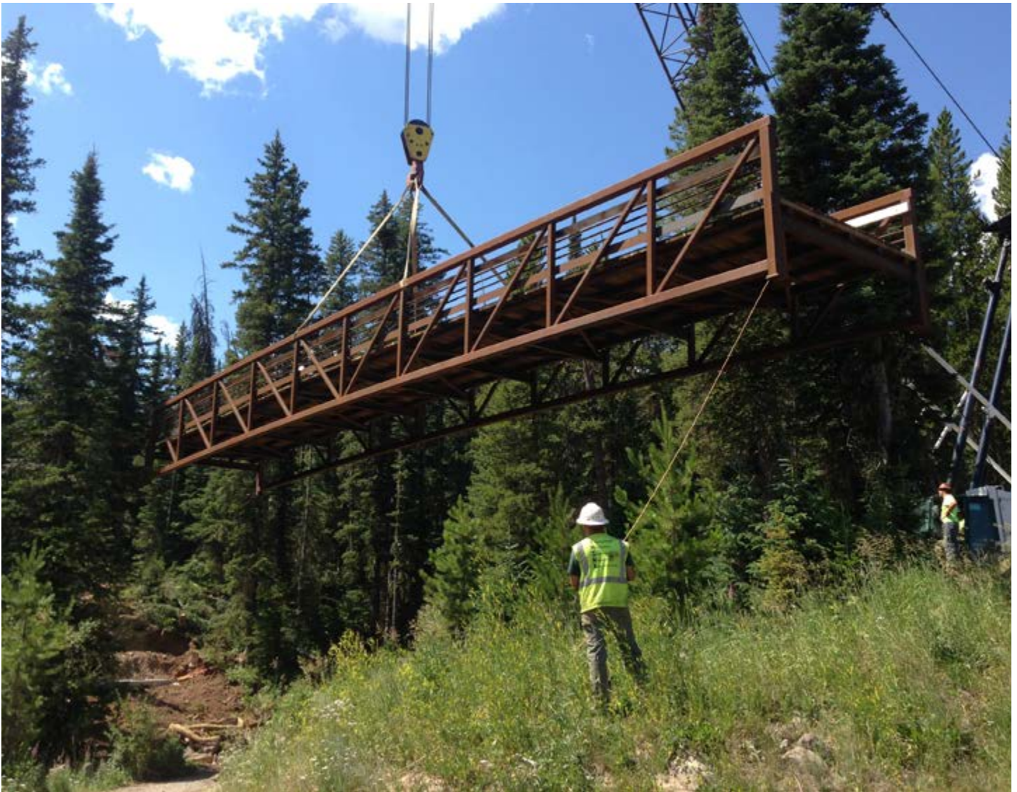
Blackmore Creek bridge installation in the Northern Region. USDA Forest Service photo.
