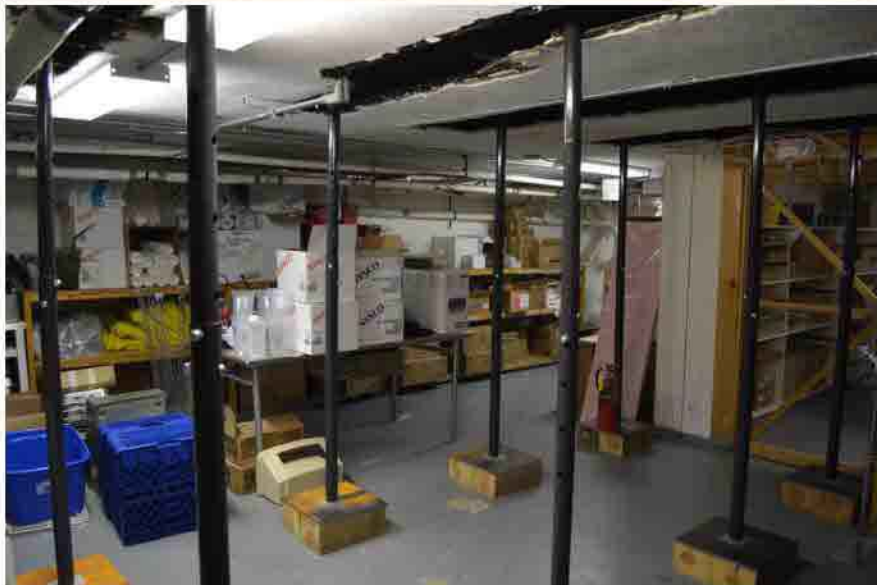
Figure 8. Example of the neglect of a property which causes its deterioration.
