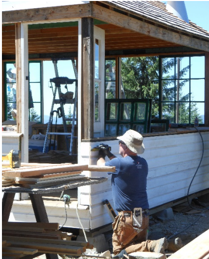
Lutherhaven volunteer applies his carpentry skills to the Spyglass ground house restoration project in July 2017. Forest Service photo by Barbara Hansen.
