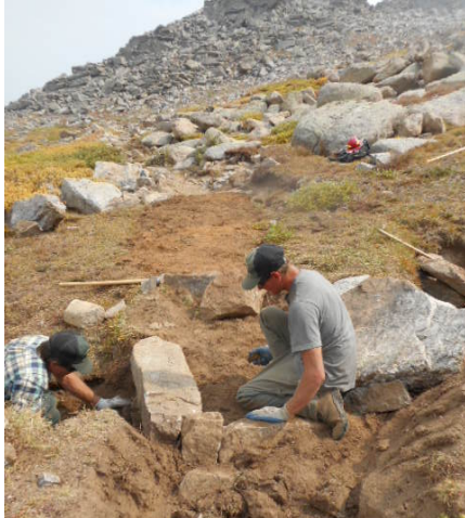
Quentin Degering instructs a Student Conservation Association Intern on the proper placement and technique of installing a culvert during the 2017 Bears Ears Blasting Project. Forest Service photo by Callie Domek.
