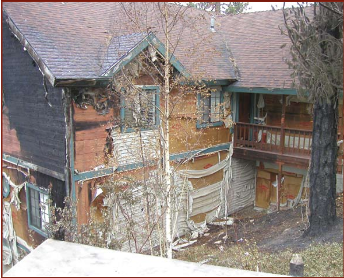
Figure 32. Home at 26150 Walnut Hills Dr. Thermal exposure from the destroyed home at 26142 contributed to the vinyl sloughing off. Surface fire burned the vinyl siding and under-layment on the northwest side (left) and worked its way up the wall burning the wood siding. Blackened asphalt shingles in the roof valley (center top) are from accumulated needles that burned.
