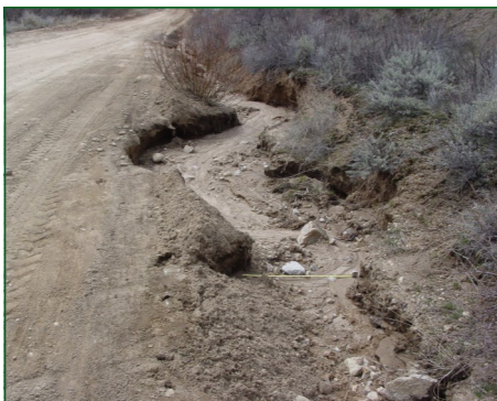
Road erosion and runoff produces fine sediment, contributing to increased sediment yields.
