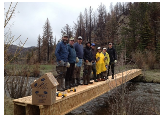
A crew constructed a sampling platform spanning the Poudre to monitor the effects of the High Park burn on stream sedimentation and water quality.
