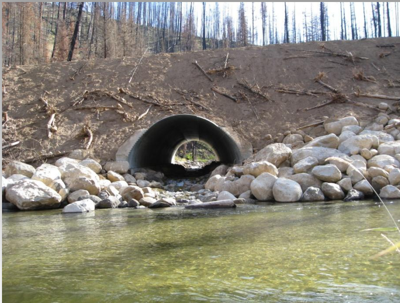
Goat Creek culvert after restoration; new aquatic organism passage (AOP), Payette NF
