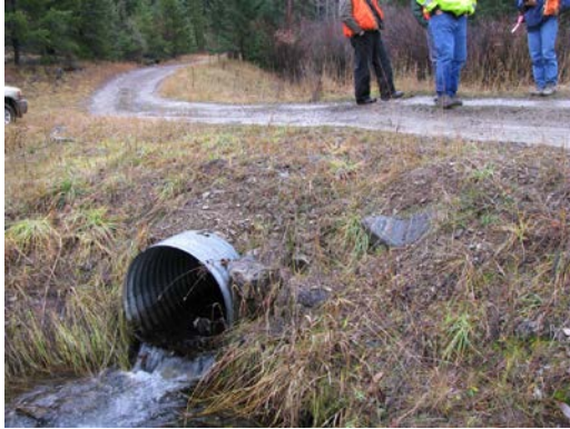
Figure 2: Undersized culvert will be replaced to accommodate fish passage and stream channel function.
