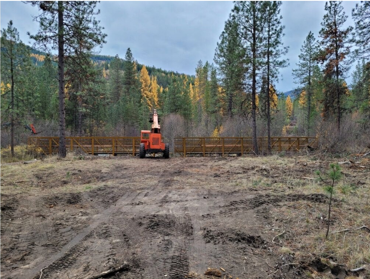
Contractor uses large construction forklifts to align and assemble the new multi-piece trail bridge over Sherman Creek.
