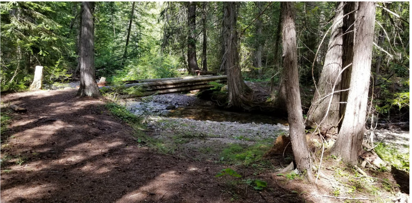
Hoodoo Canyon trail bridge over Deadman Creek that was replaced to move abutments out of stream channel and elevate the stringers to accommodate a 100-year flood event.
