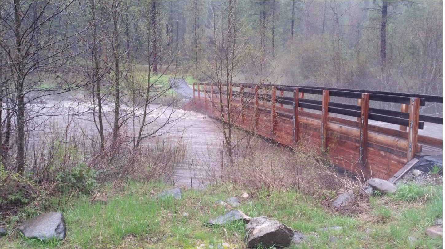
Original Canyon Creek trail bridge over Sherman Creek during high water in May 2017. Abutments were located within the river channel and high water would hit the north end stringers and undermine the north end abutment.
