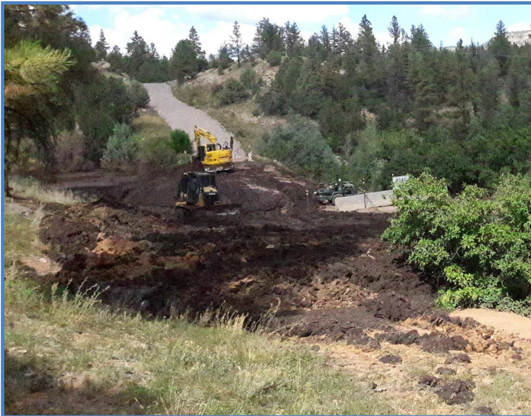
Removing debris and replacing a culvert plugged by debris flows following thr Venado Wildfire. Plugging of the culvert threatened to cause the 30" high road fill to fail, which would have resulted in massive sediment inout into the Rio Guadalupe. September 2019
