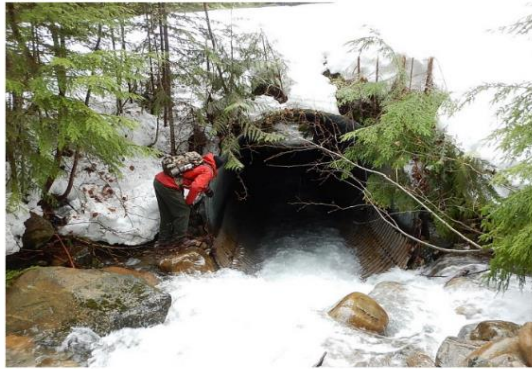
Undersized culvert inlet pre-replacement.
