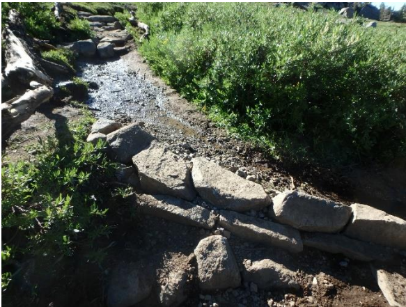
American Conservation Experience crew repaired water bars on the well-used trail to Winnemucca Lake. Photo by Chip Morrill
