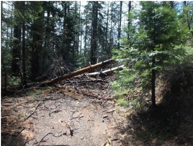
American Conservation Experience crew cleared numerous trees to help make the Gold Note OHV trail system accessible to the public. Photo by Chip Morrill
