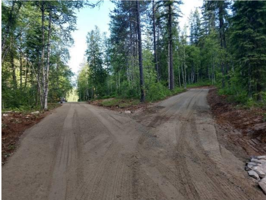
Figure 7: Main Solomon Lake Campground road with campground loop to the right. Subsequent work by rec crew installed parking blocks and stabilization material.
