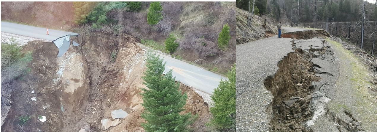
Storm damaged roads in the Cornerstone area of the Eldorado National Forest.
