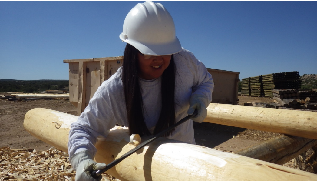
Image 2: Jemez Crew member practices her hand viga peeling skills at a visit to the Walatowa Timber Initiative wood processing plant.
