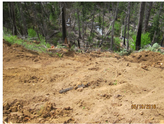
Weight of equipment initiated additional slides. Only a matter of time before entire road failed.
