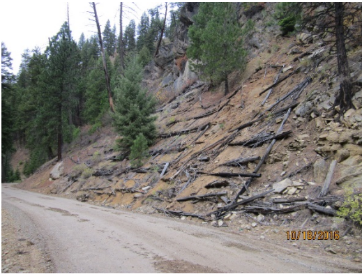
Before – Attempts to use logs in the past have failed.
