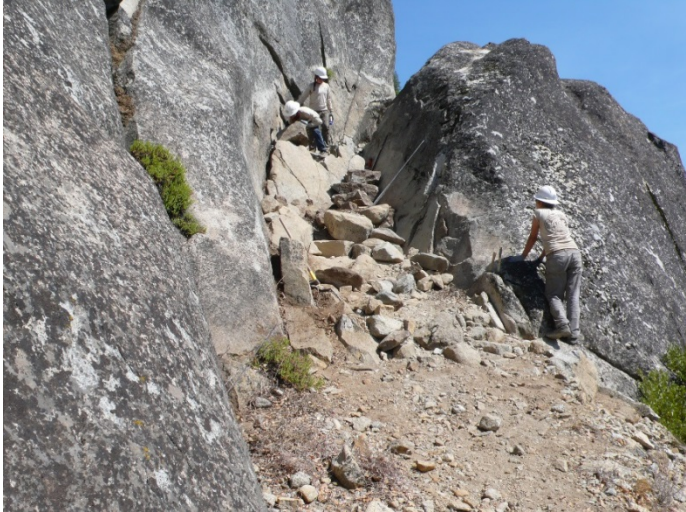
ACE crew installing rock steps on Salt Springs trail. Photo by USFS
