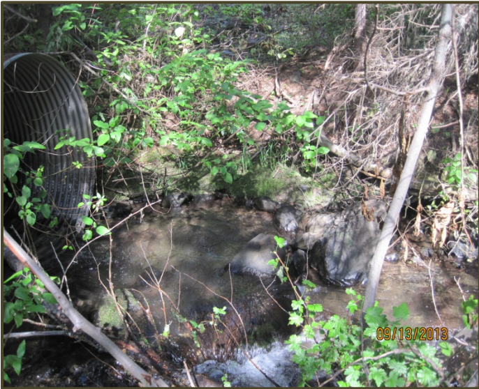
Before photos of an Aquatic Organism Passage construction at Ant Basin Creek
