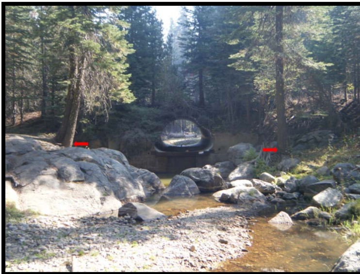
Culverts can greatly reduce the velocity of stream flow and limit the movement of animals such as frogs and fish. Photo represents pre-treatment. Photo by USFS.
