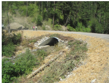
Figure 11: McCabe Creek aquatic organism passage. Left photo = Before. Right photo = After aquatic passage culvert installed.
