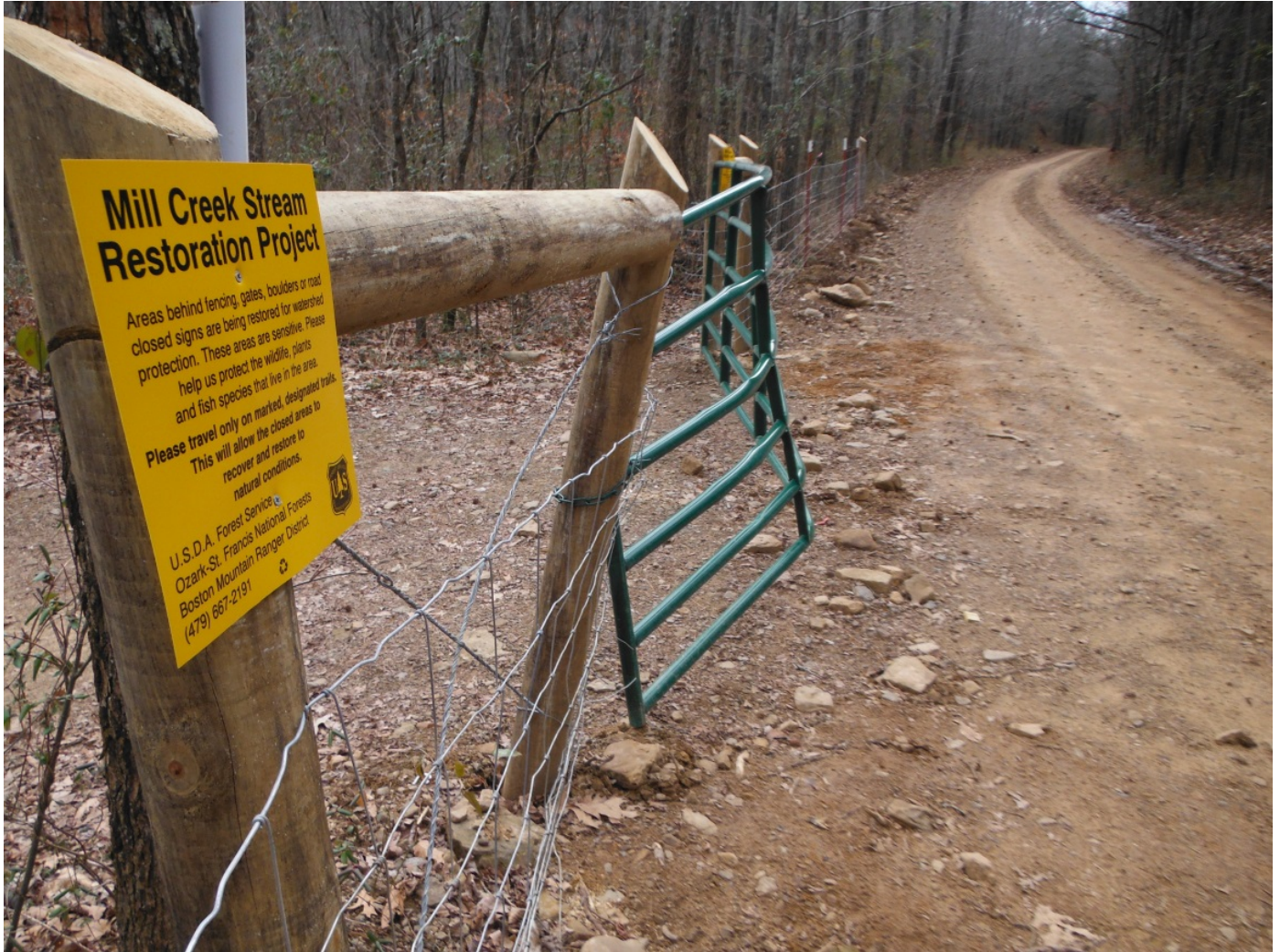
Figure 3. Gate damaged at Mill Creek area.
