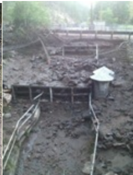
Monroe Diversion damaged by flooding
