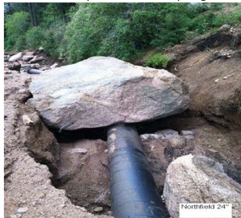
Damage to water delivery infrastructure
