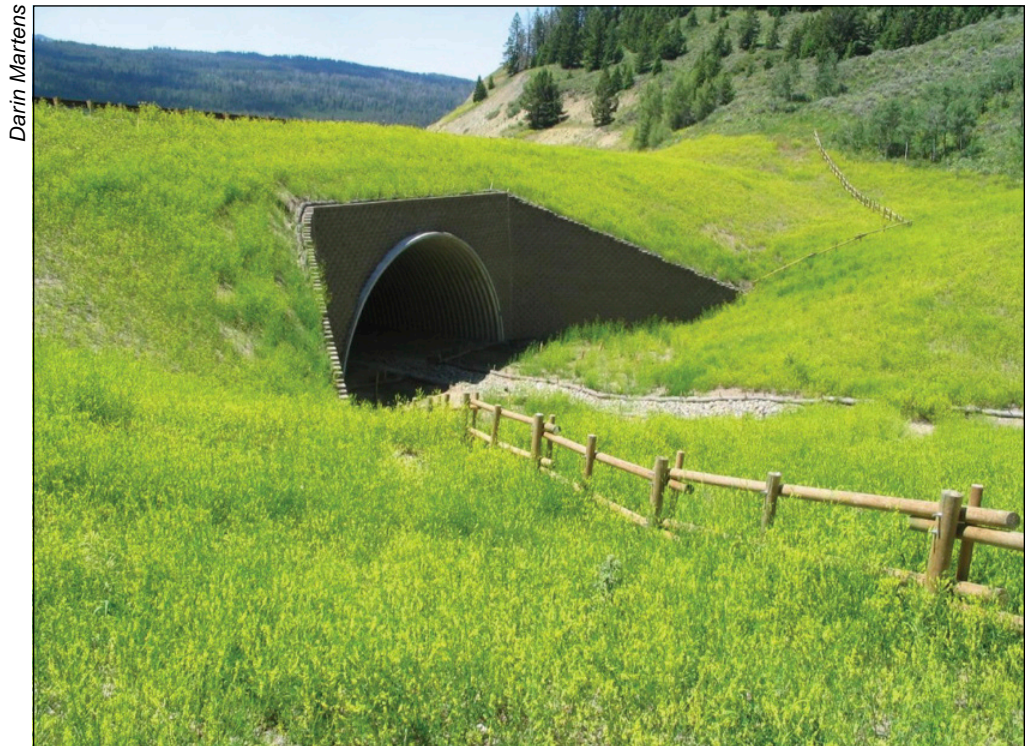
Figure 9—Togwotee Corridor reconstruction, 50' diameter arch wildlife crossing structure during the flowering of yellow sweet clover ( Melilotus officinalis ).
