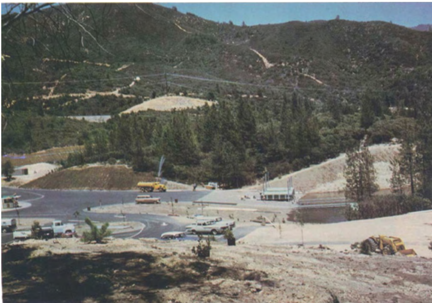
Figure 16 —Oak Bottom Beach, Whiskeytown Reservoir, under construction in 1964. Notice the tractor trails on the background hill.
