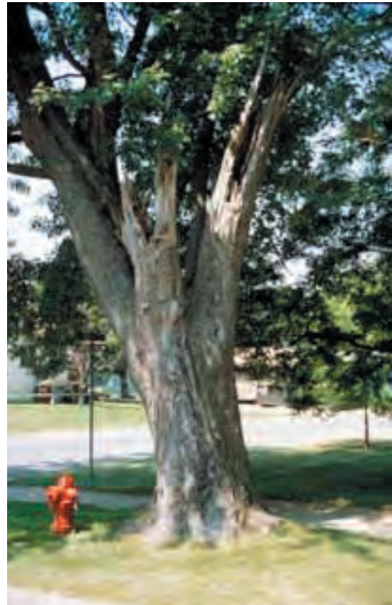
Figure 5.1. This tree was previously topped, and extensive wood decay has developed as a result. Two major branches have already failed. This tree will continue to decline at a rapid rate and should be removed.
