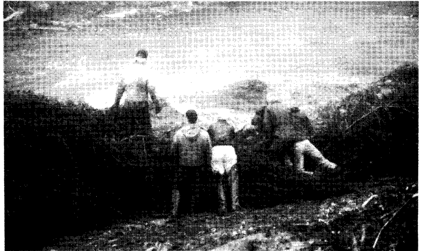
The 15- to 20-foot cedar trees were installed in an overlapped fashion and anchored with a duckbill anchor four- to five-feet into the bank.
