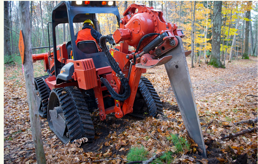
The vibratory plow blade cuts narrow trenches 5 feet deep to separate underground root systems, preventing further spread of the oak wilt fungus to uninfected trees.
