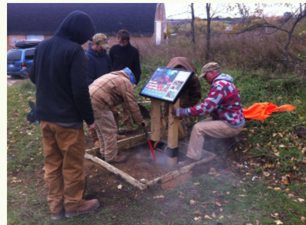
Grand Traverse Conservation District Employees and SEEDS crew members work together to install a boot brush station at Historic Barns Park in Traverse City Commons. Patrons use this station to clean seeds, mud, and other plant material from their boots, in order to prevent them from spreading invasive plants.
