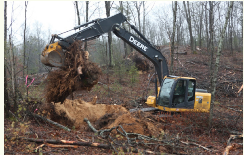
Pulling stumps of newly infected trees prevents the oak wilt fungus from moving through roots to other trees.
