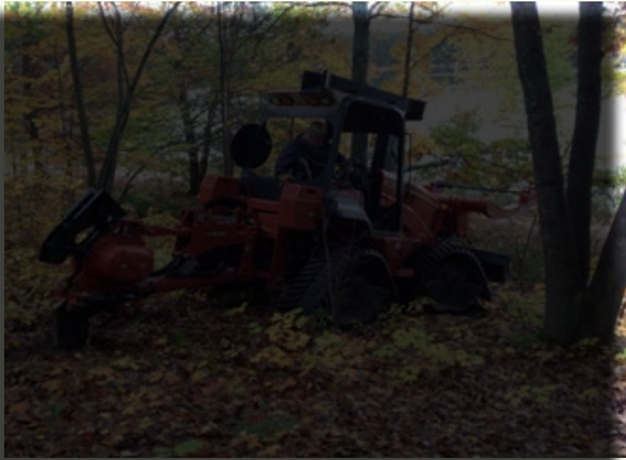
A Department of Natural Resources employee installs root graft barriers with a vibratory plow.
