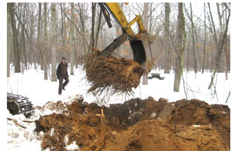
Staff use a clamshell excavator to remove the stump of an infected tree and cut root grafts before fungus can move to adjacent healthy trees.
