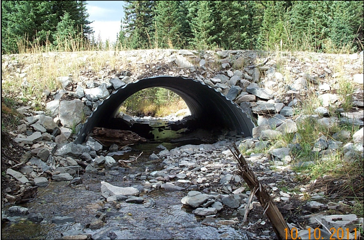
Figure 2. Culvert built to mimic natural stream reaches. The stream flow and substrate within the culvert remains similar to that of the adjacent upstream and downstream reaches. In this case fish passage should be assumed.
