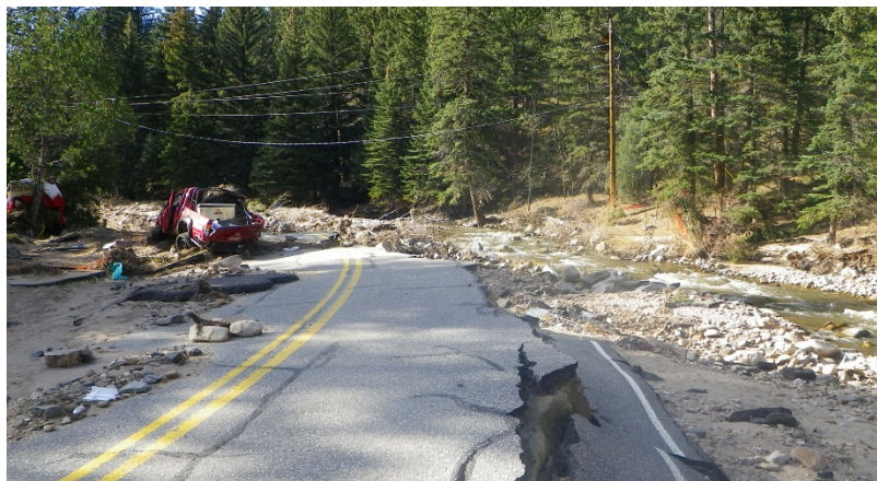
Figure 1: Flood damage in Glen Haven, Colorado (10/18/2013).
