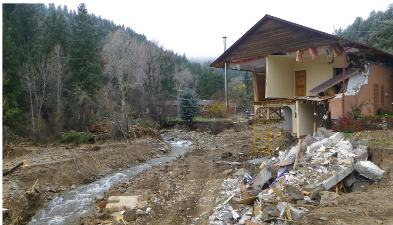
Figure 3: Flood impacts in Jamestown, Colorado (10/29/2013).
