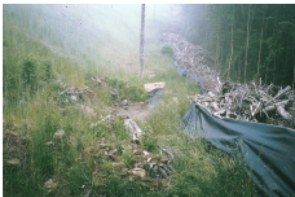
Figure 8. Geotextile lined slash windrow at the fill slope toe to detain surface flows from the road and trap sediment.
