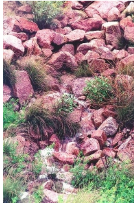
Figure 10. Rock riprap protection for a cross drain outflow on the fill slope.
