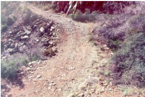
Figure 3. View of porous fill looking up the road. Note the retaining walls on each shoulder.
