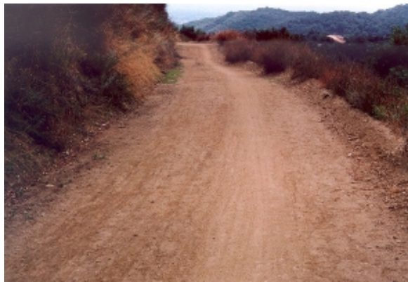
Figure 16. Berm on downhill shoulder to protect steep fill slope from surface flows.
