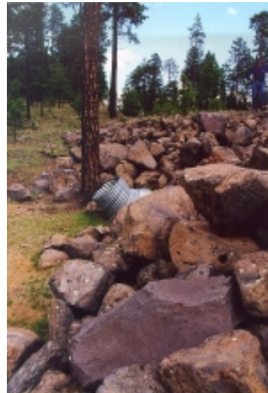
Figure 17. Raised inlets on road stream crossing to pond water and preserve sediment.
