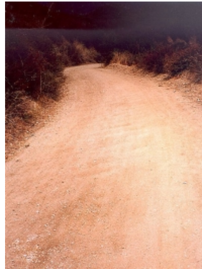
Figure A10. In sloped traveled way with large berm on outside shoulder. Note the existence of rills running perpendicular to road center line even after surface blading.
