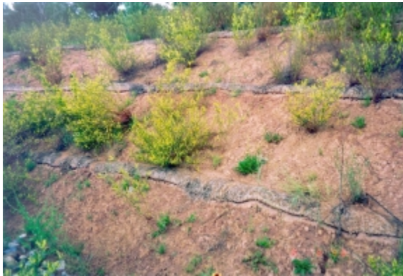
Figure 7. Rolled straw bales placed on back slope to break up surface water concentration and reduce erosion.
