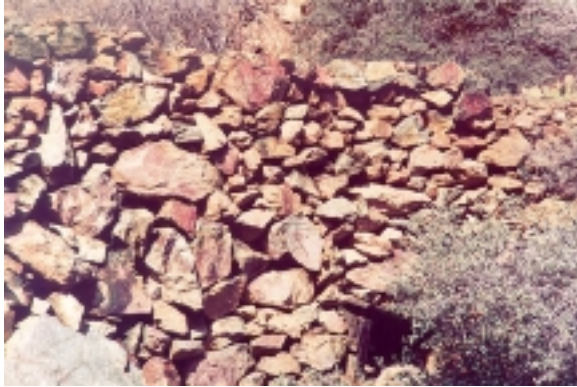
Figure 2. Downstream view of porous fill road-stream crossing. Note the square culvert made of rough sawn dimension lumber (non-functional). Stream is flowing under culvert.
