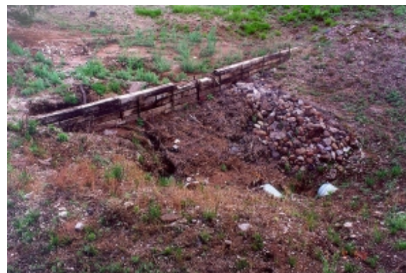
Figure 19. Used railroad tie structure to pond water and preserve sediment upstream of a road stream crossing.
