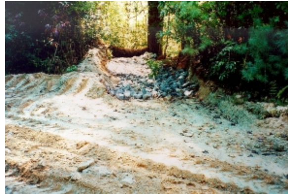
Figure A16. Rock armor and silt fence at lead out ditch outflow to reduce erosion and sedimentation.
