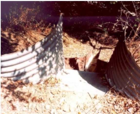
Figure 13. Fill slope protected by corrugated sheet metal flume at a cross drain outflow.
