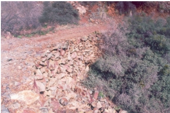
Figure 4. View looking down the road at the downstream porous fill retaining wall.
