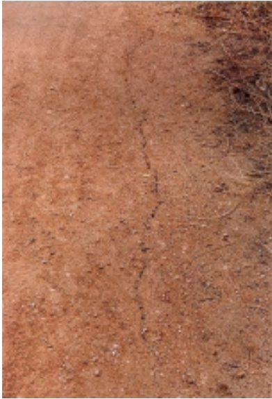
Figure A12. Tension cracks in traveled way surface made worse by weight of berm on downhill shoulder.
