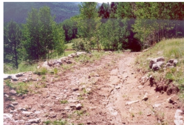
Figure A3. Low volume, single lane, native surfaced logging road in northern New Mexico.
