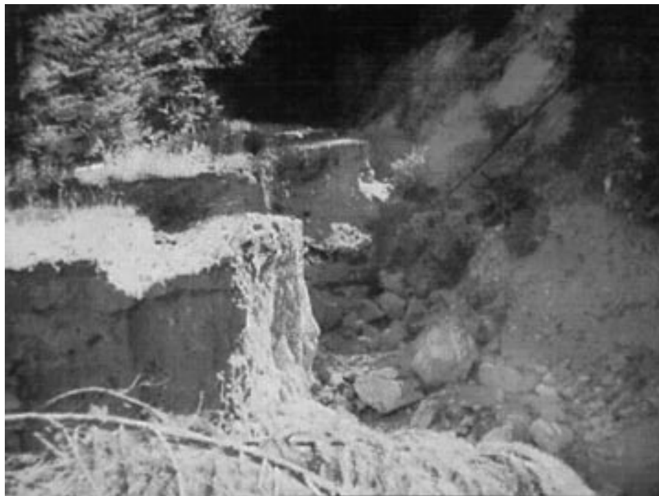
Figure 5—Severe gullying at K-Creek flood-assessment site.
